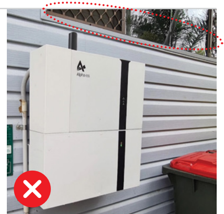
Figure 6.2: In this example the window above the battery system vents a habitable room and is located within the exclusion zone outlined in Figure 6.1.
