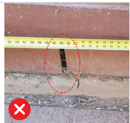
Figure 1.3 The presence of a penetration greater than 5mm in diameter through the non-combustible barrier to a habitable room and within 600mm of the left edge of the battery system is non-compliant unless sealed with fire-retardant material.
