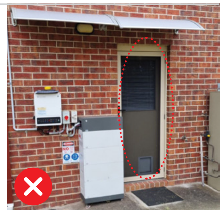
Figure 7.3: This battery system is non-compliant as it has been installed too close to an entry or doorway.
