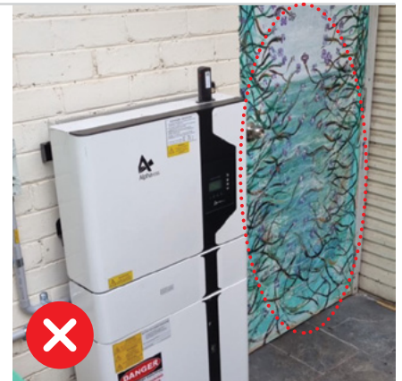
Figure 7.2: This battery system is non-compliant as it has been installed too close to an entry or doorway.
